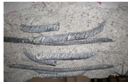
Figure 6. Detachment of the concrete cover of the specimen J05 (Realfonzo et al. 2014).
